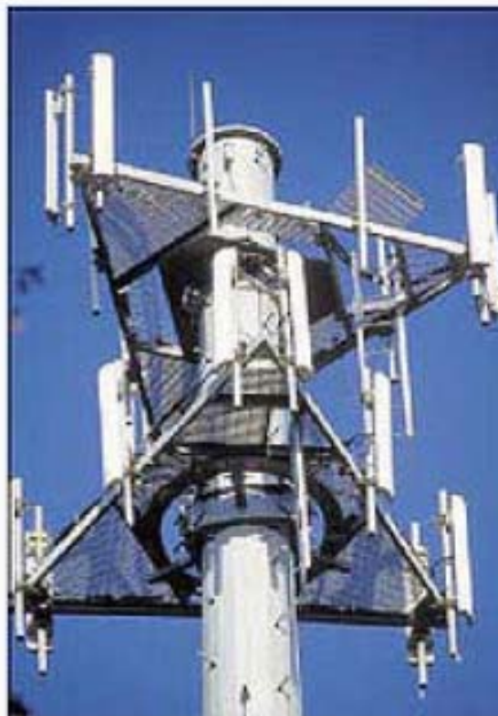
Cell phone base station antennas
